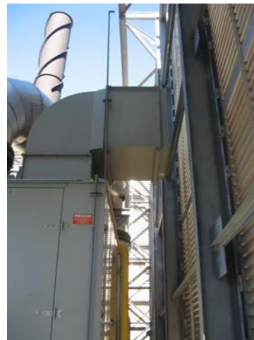
Inlet vent and exhaust stack
