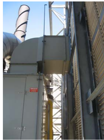
Inlet vent and exhaust stack
