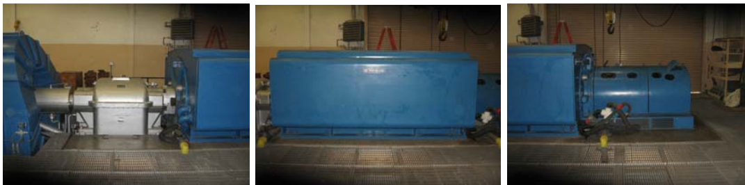
Gearbox, generator, and alternator sections
