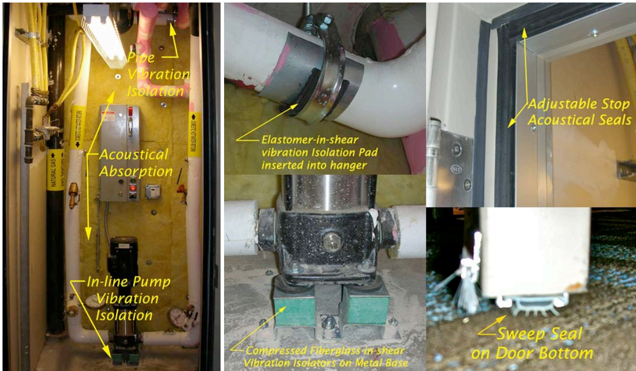
Figure 6. As-installed modification illustrations: Pump closet view with acoustical absorption (left), pump and pipe vibration isolators (center) and door head, jamb and threshold seals (right).
