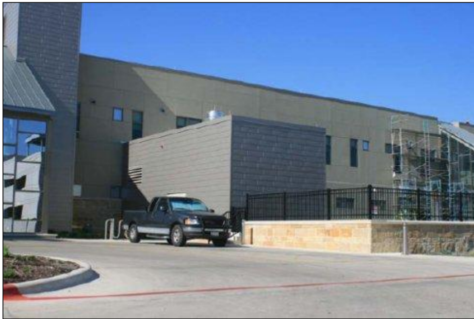
Figure 7. The location of new underground MRI addition after construction. The roof of the addition with fence railing on top is in the foreground (center right).
