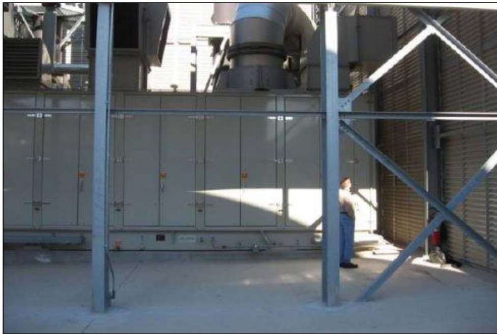
Figure 2. Gas turbine generator enclosure inside the plant. The grout-filled floor cavity is in the portion below the door panels.
