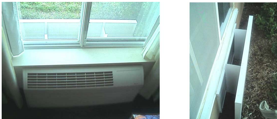
Figure 6: inside (left) and outside (right) views of typical air conditioner with baffle
